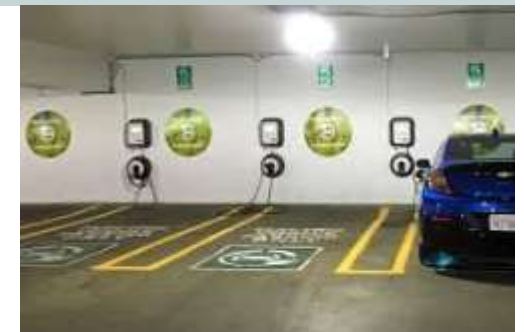
Car park provision of slow chargers
